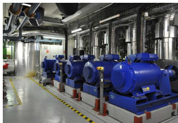
Example of a heat exchanger in the CLIMESPACE "Canada" district cooling production centre in Paris. This unit uses river water from the Seine in the cooling production cycle. (Photo courtesy of John Dulac).
