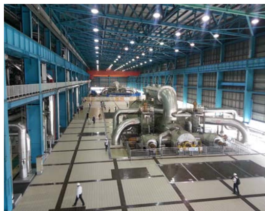
Steam turbines at Waigaoqiao, Shanghai. (Photo courtesy of the CCC TCP)
